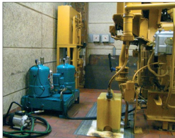
E.ON Danmark A/S, Caterpillar Gas Engine and the CJC™ Fine Filters 2 x HDU 27/27 PV
