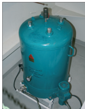
CJC™ Fine Filter HDU 427/81 installed in the engine room
