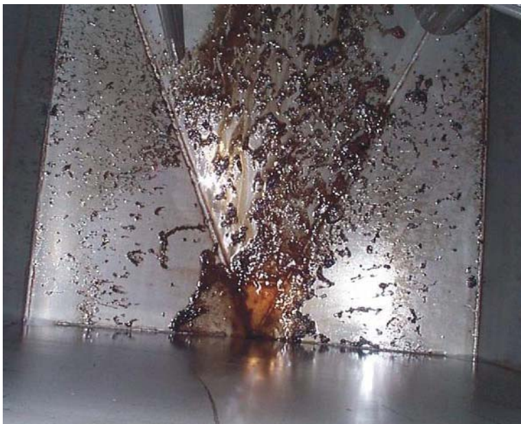
Drained oil tank without offline filtration
