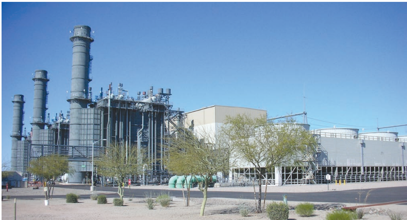
1. New Harquahala Generating Co is an 1100-MW plant with three 1 × 1 combined cycles powered by Siemens Energy SGT6-6000G (W501G) engines
