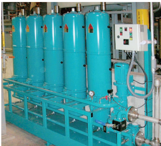
6. Steam turbine lube-oil conditioning system has five independent modules operating in parallel. Each has multiple filter inserts and a coalescer element
