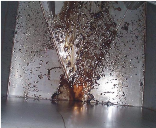
Drained oil tank with varnish and particles
