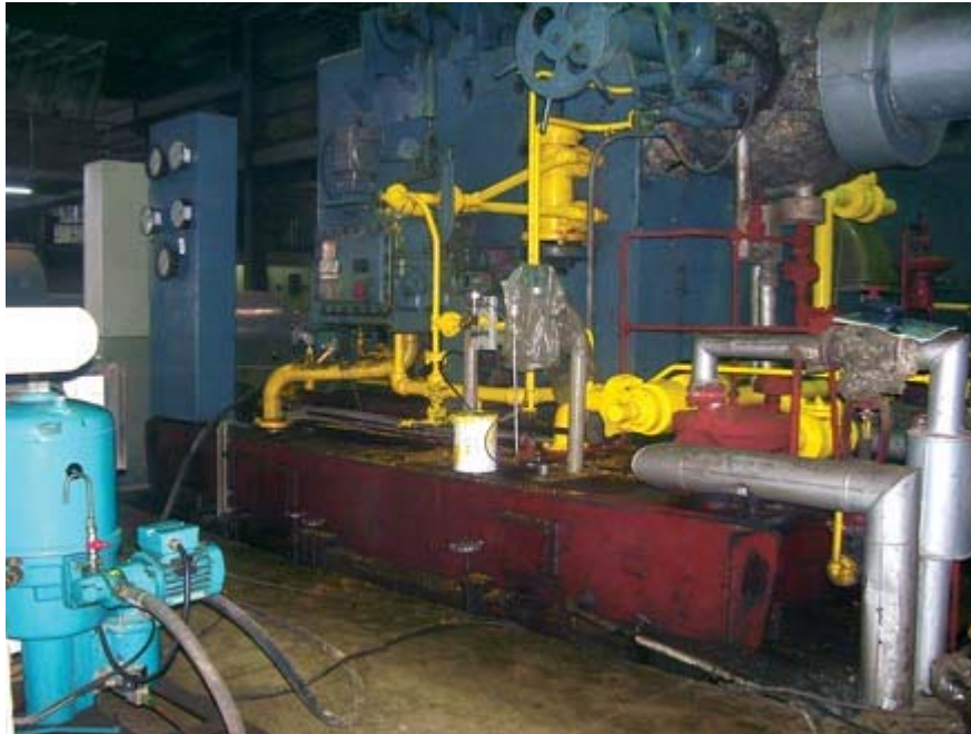
Figure 3. The water separator unit was installed adjacent to the 5-megawatt Turbodyne steam turbine.
