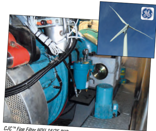
CJC™ Fine Filter HDU 15/25 PV2 installed at North American Wind Research and Training Center
