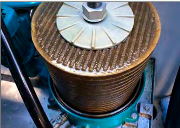
Even a large oil filter is drained within minutes. Installation at RWE Wind Services
