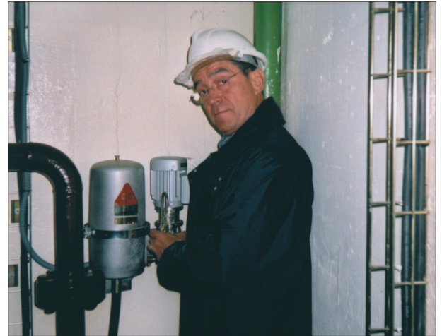
Mr. Jesus Javier Moises in the hydro-electric generation station, next to the CJC™ LG 15/25 L Fine Filter.
